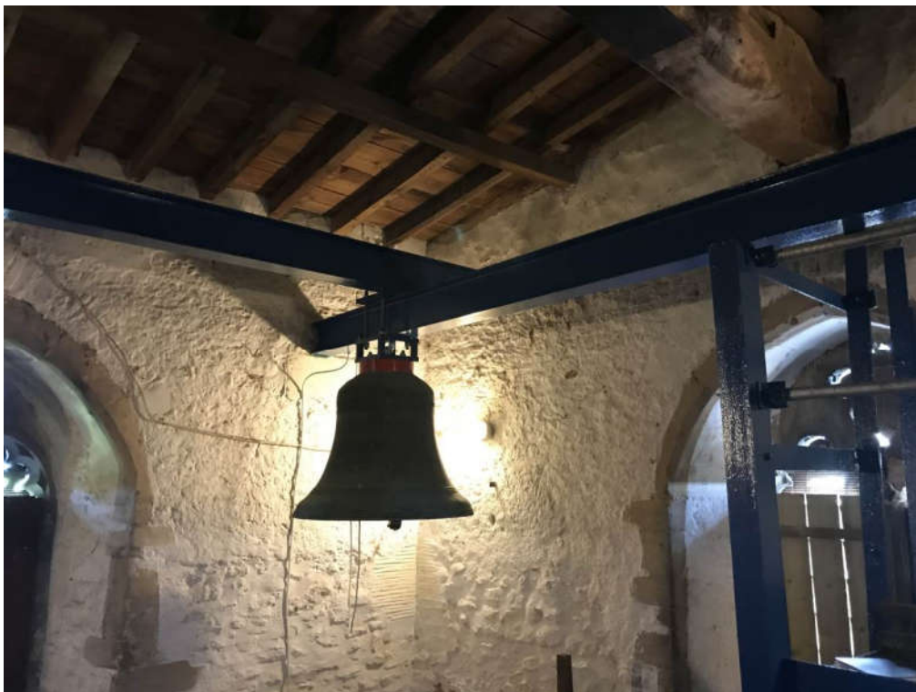
Photograph 10 – 'Modern' steelwork supporting bells
