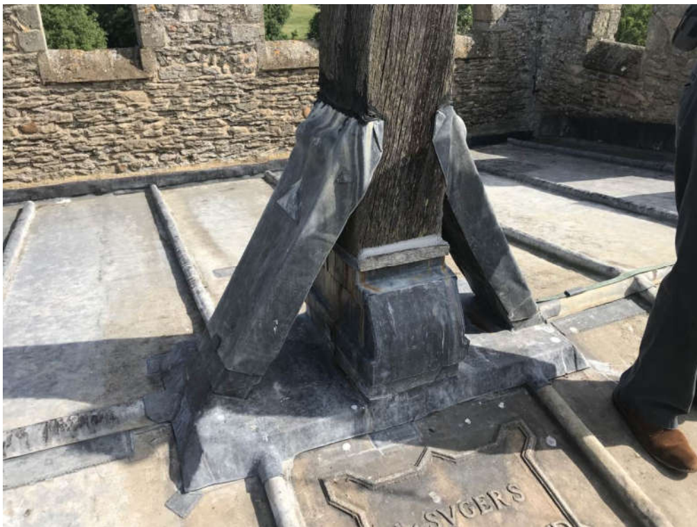
Photograph 4 – Poor leadwork details around existing post
